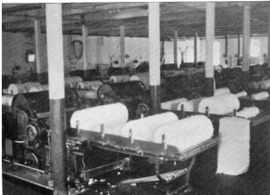
FIG. 12.—VIEW OF ABOVE PICKER ROOM AFTER INSTALLATION OF INDIVIDUAL ELECTRIC DRIVE
