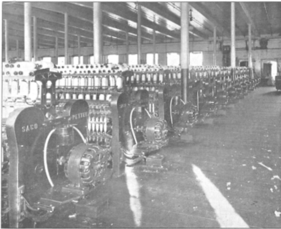
FIG. 10.—SPINNING FRAMES AT THE CHICOPEE MFG. CO. MILL, CHICOPEE FALLS, MASS. DRIVEN BY WESTINGHOUSE TEXTILE TYPE MOTORS
