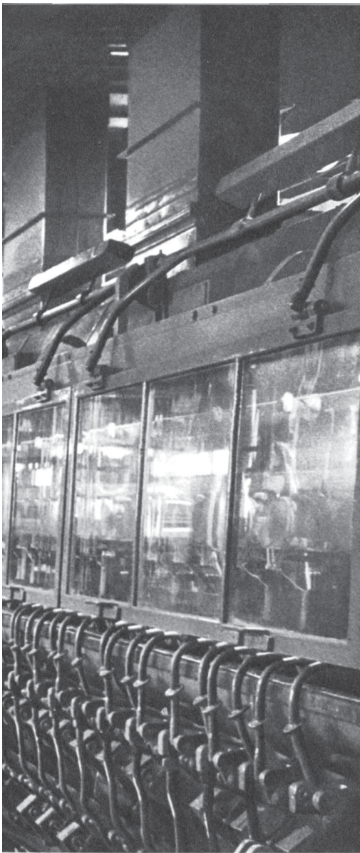
The staple fibre spinning room of the Nanking Chemical Fibre Factory, one of those built this year
