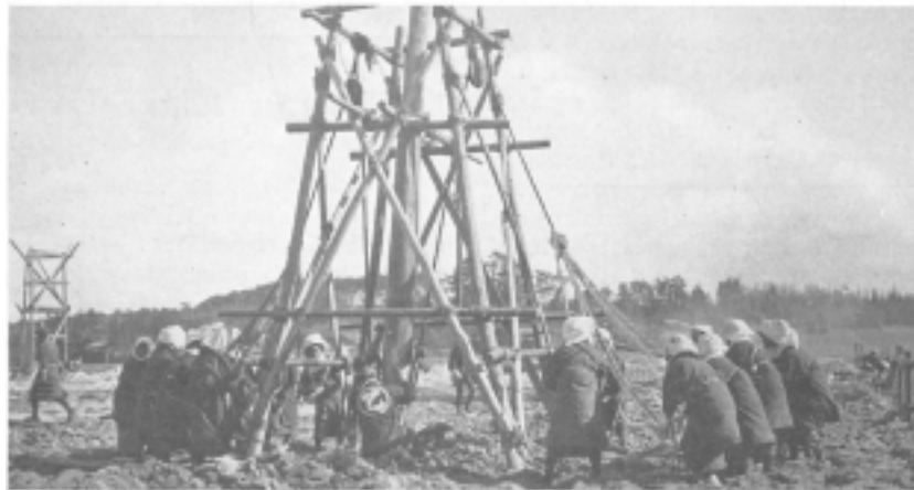
Tamping ground for pier foundations of a Japanese mill—Aichi Orimono Mill, Nagoya, Japan
